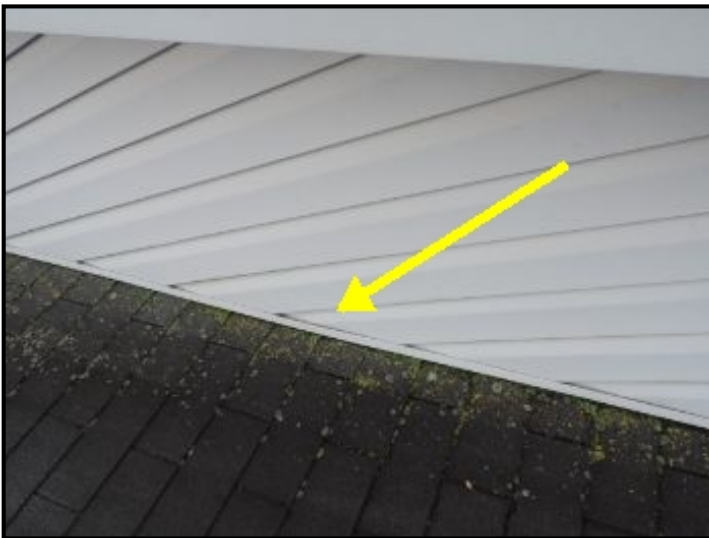
moss on roof
